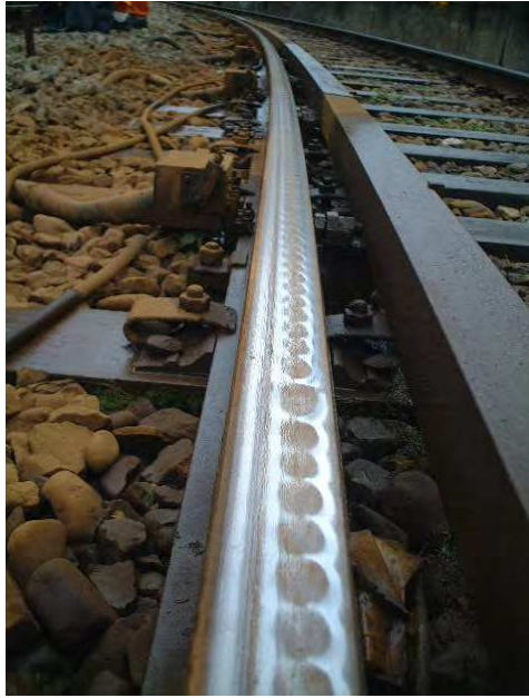
Fig. 2. Example of rail corrugation
