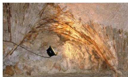
Fig. 2. Reed centring in the Roman concrete vaults beneath the Villa Medici, Rome. Reproduced by permission of Matthew Bronski
