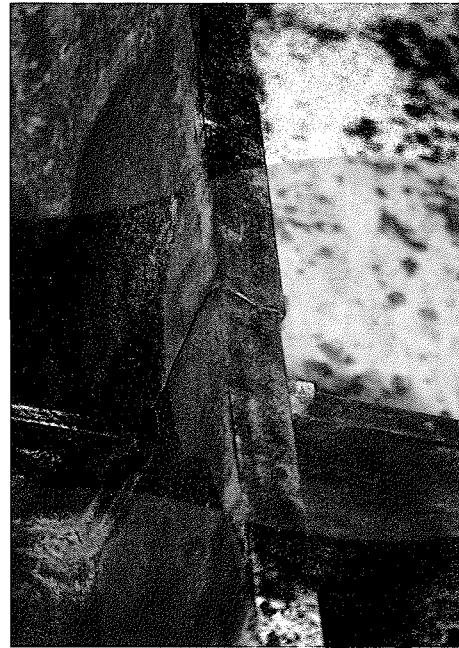
Fig. 42. Moment resisting frame under construction: close-up view of a beam-column connection damaged by column flange fracture at the level of the column web stiffener (left) and beam's lower flange (right).
