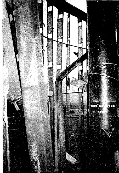
Fig. 2. Kaiser Permanente Hospital: buckled double angle chevron bracing in penthouse.
