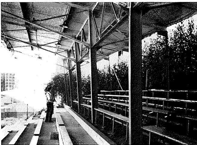
Fig. 9. Roof structure covering the bleachers of the football field at the California State University at Northridge: cantilevered steel frames.
