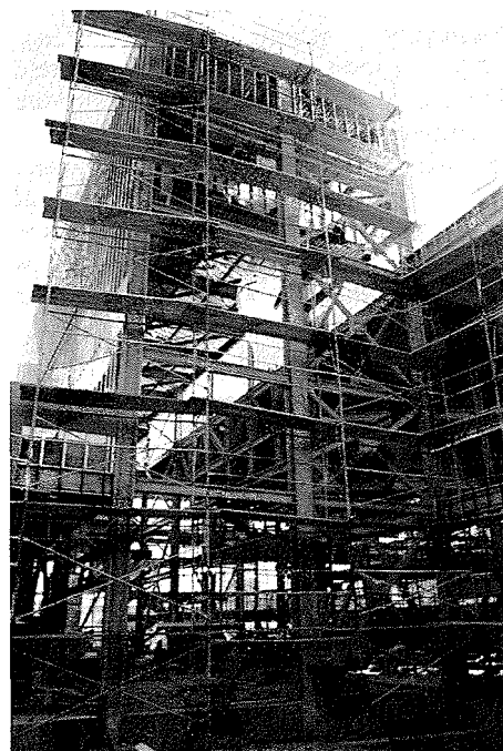
Fig. 7. Student Union Building at the California State University at Northridge: exterior view of building bracing system.
