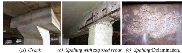
Figure 1. This paper only concerns the crack(a), spalling with exposed rebar(b), and pure spalling(c) three kinds of concrete flaws. The condition states of these flaws consist of CS1 (good), CS2 (fair), CS3 (poor), and CS4 (severe) four degrees.
