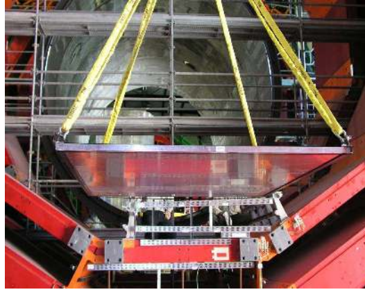
Figure 26: A fully assembled panel of HO being mounted on one of the outer rings (ring +2) of the magnet yoke.
